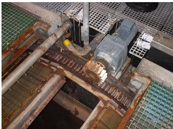
Fig. 9. Corrosion of rotating screens.
